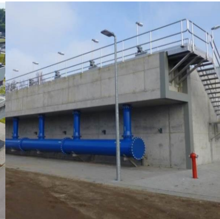
The 1-STEP filter at the Horstermeer wastewater treatment plant
