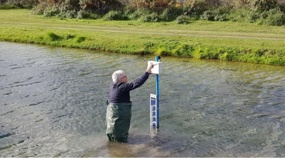
Installing water level sensor using LPWAN.
