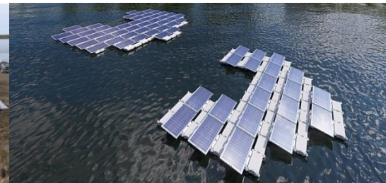
Floating solar panels
